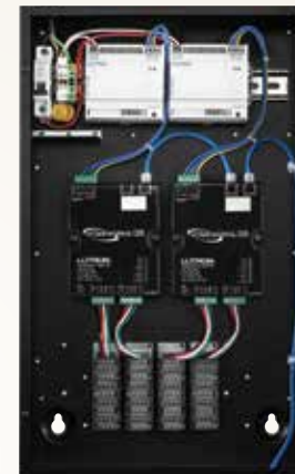
21" Low Voltage Enclosure
